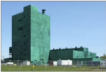
Figure 17. C-340 Metals Complex with transite siding that is sealed to stabilize hazardous and radioactive materials during demolition
