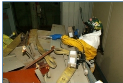
Figure 22. Deactivation radiation screening
