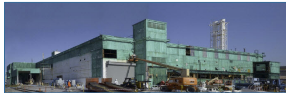
Figure 21. C-410 & C-420 Complex
